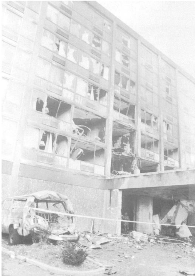
FIG. 1—Front of building after the fire was extinguished. Note that the burn pattern from the fuel/air fireball extends to the top of the building.
